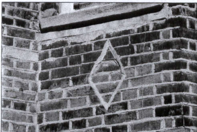
● Poor pointing spoiling brick details
