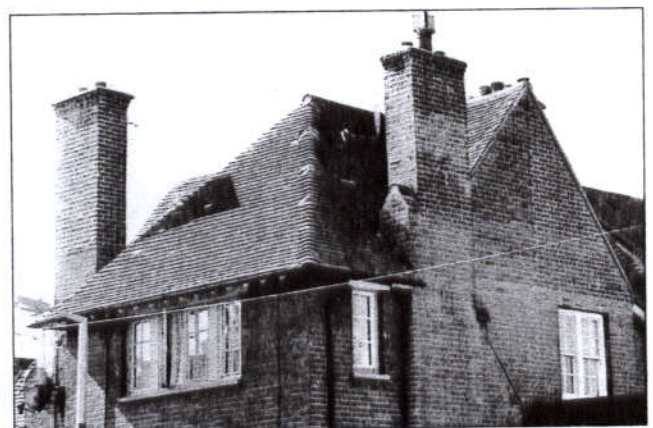
● Dramatic roofline with imposing Tudor style chimneys but the poor pointing detracts from the effect
