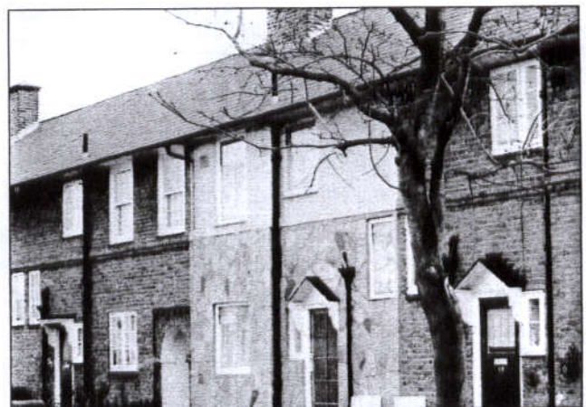
● The uniform character of this row is undermined by cladding, painted brickwork and replacement windows and doors
