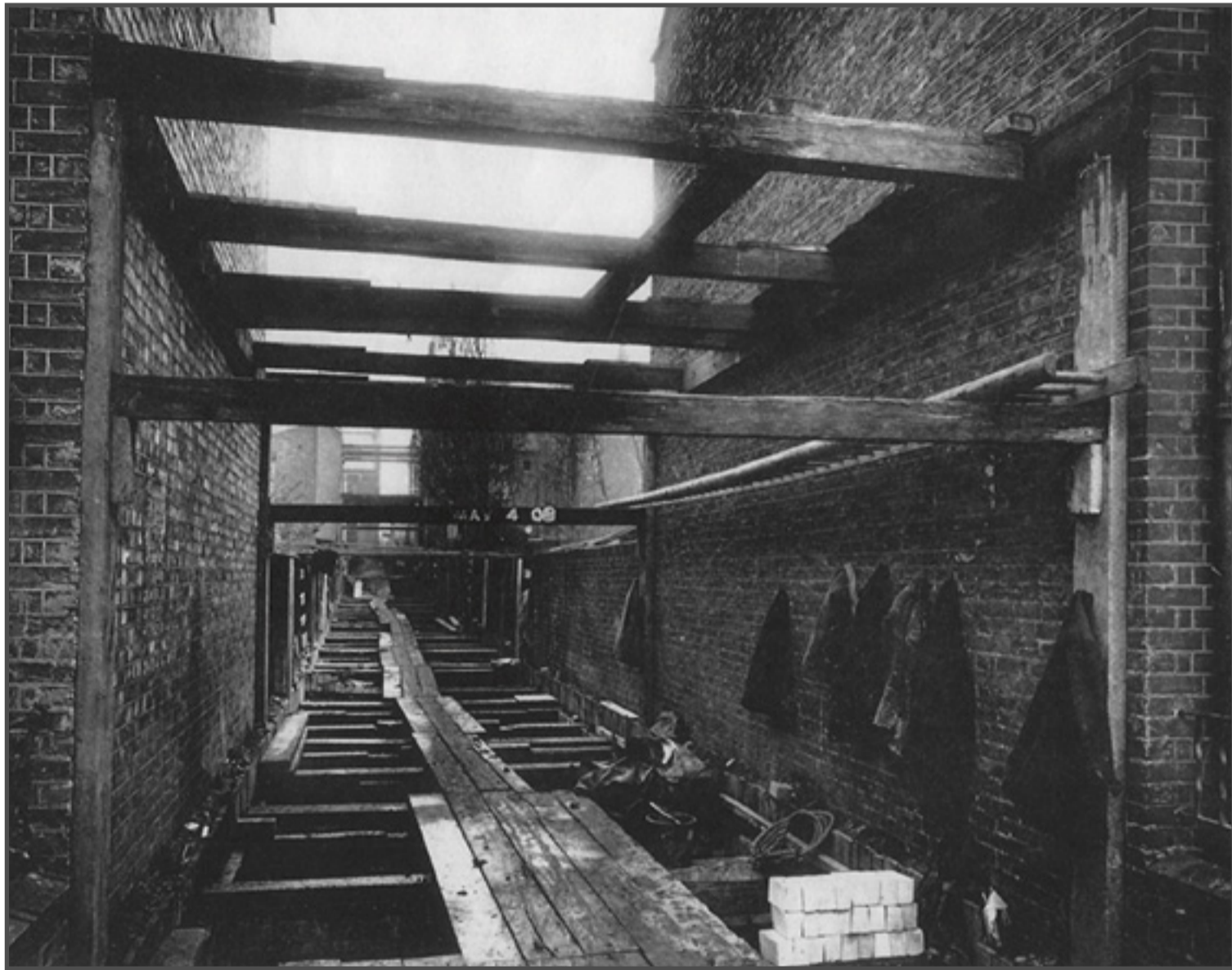
Up-grading works to the sewers, Fairfax Road, 1903. Courtesy of Kevin Lincoln, Haringey Council
