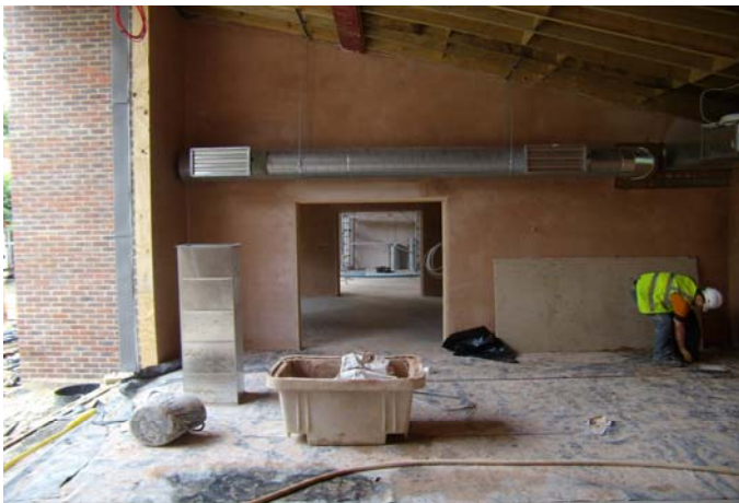
Block C, single storey building, which will be occupied by reception children in September.
